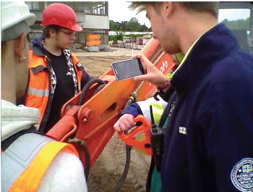
Figure 6. Field case study at BauABC: The apprentices show a close up of the joints and cylinders to the instructor remotely via SoAR, and the instructor notices that the cylinder is causing the noise. After inspecting under the cylinder, he instructs the apprentices to lubricate it again.
